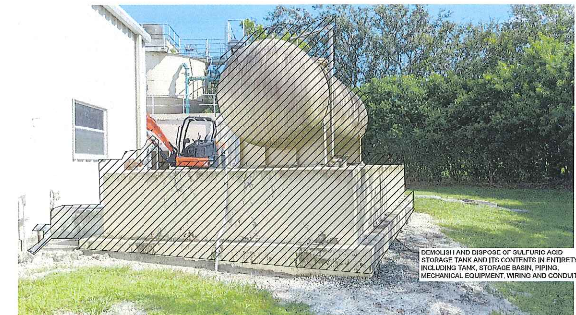
V PHOTO FILE: SULFURIC ACID STORAGE TANK-3
