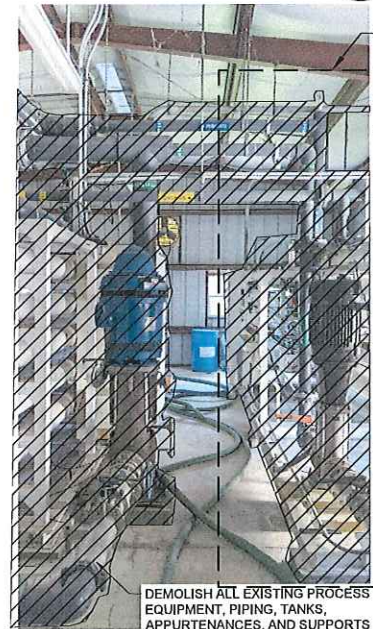
BB PHOTO FILE: RO FILTRATION BUILDING INTERIOR-1-3
