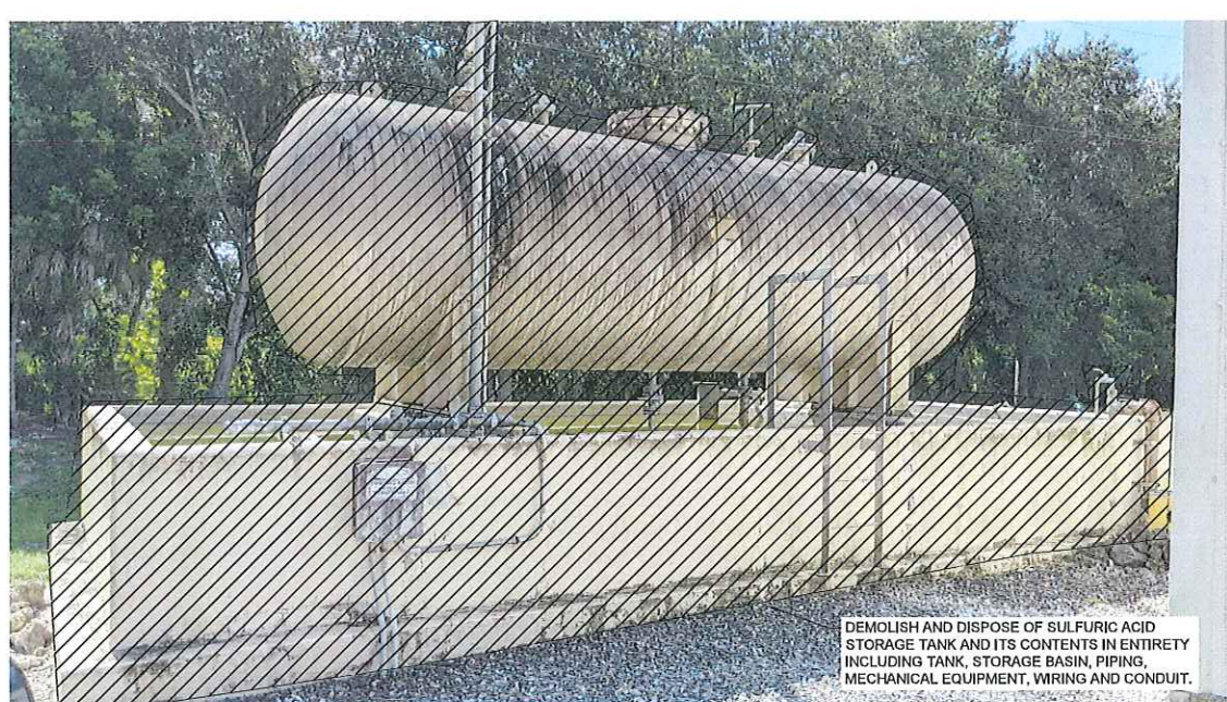
U PHOTO FILE: SULFURIC ACID STORAGE TANK-2
