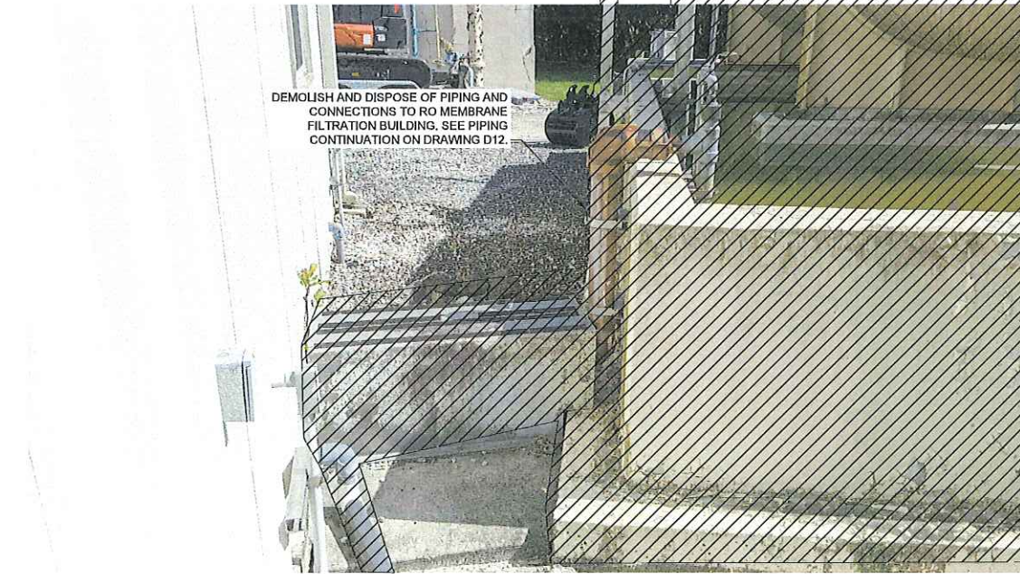
W PHOTO FILE: SULFURIC ACID STORAGE TANK-4
